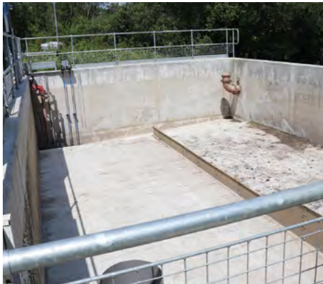
North Petherwin storm tank
