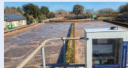
Direct N_2O monitoring equipment at our Dawlish wastewater treatment works
