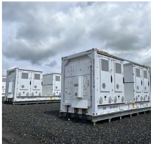
Dunfermline – Battery Energy Storage System
