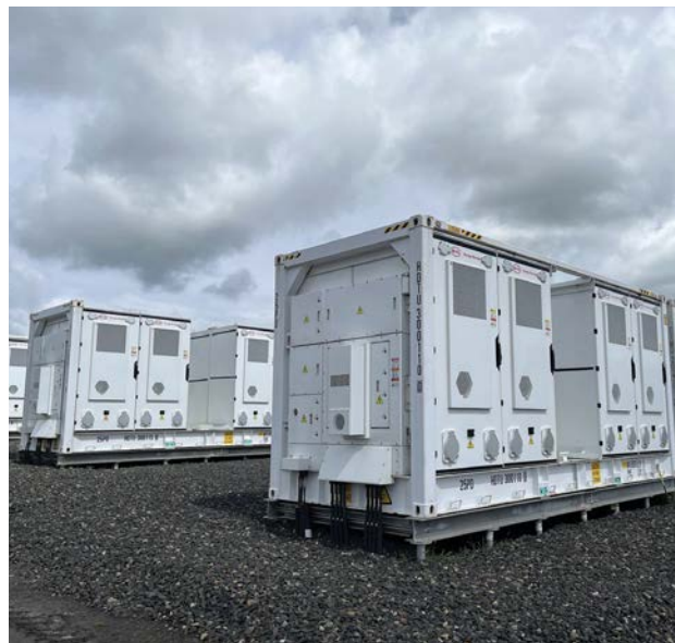
Dunfermline – Battery Energy Storage System
