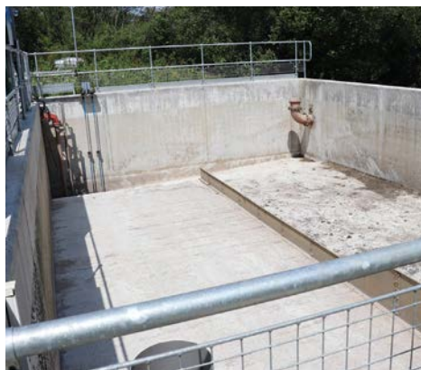
North Petherwin storm tank
