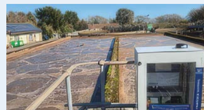
📍 Direct N 2 O monitoring equipment at our Dawlish wastewater treatment works
