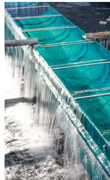
🔍 Granular Activated Carbon (GAC) at Littlehempston water treatment works
