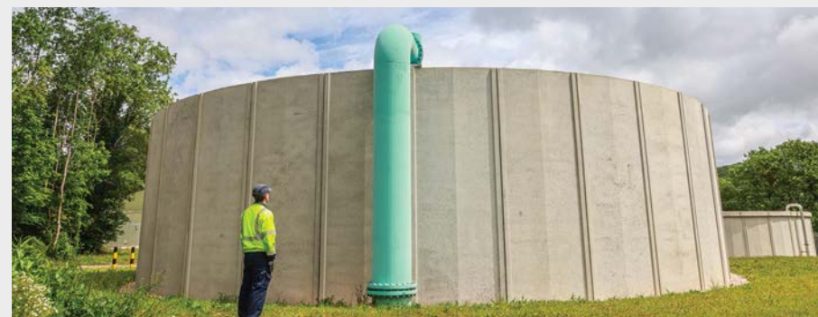
Littlehempston Water treatment works
